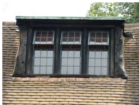
Picture 3.69 Sloping pitched roof dormer to the Tithe Barn, Old Church Lane
