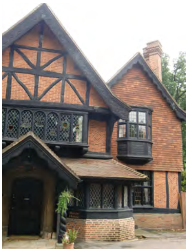
Picture 3.45 Varied roofscape, decorative mock timber framing, tile hanging and jetty overhang
