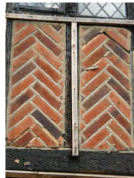
Picture 3.67 Herring bone patterns infilling mock timber framing panels on the locally listed Gate House Lodge, Old Church Lane
