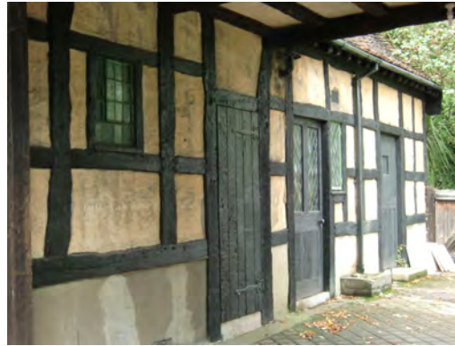
Picture 3.49 Lathe and plaster infill on wall to the grade II listed Cowman's Cottage, Old Church Lane and part of its roof over the carriage-way
