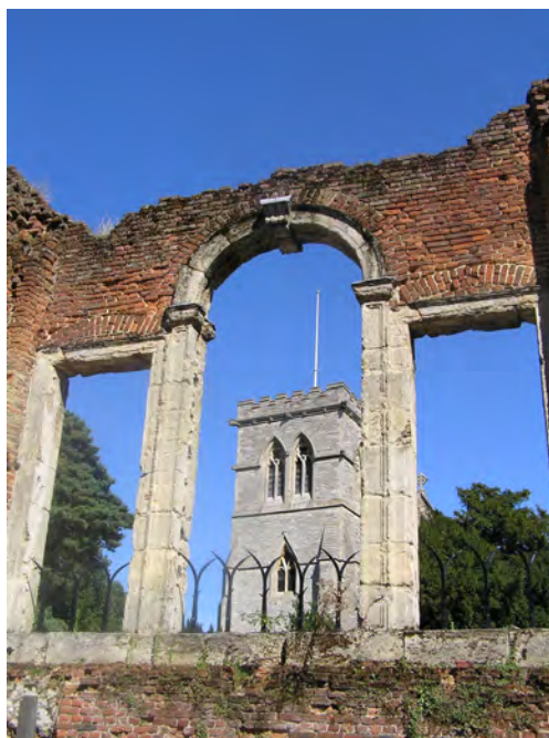
Picture 3.26 View towards the remains of a wall to the Old Stanmore Church, with the Church of St John the Evangelist behind
